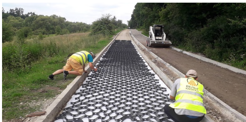
Fig. 2. Construction of the first part of the Green Line project in Ivan Pavel II Park. June 2022
