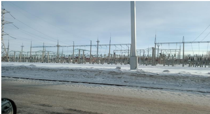
Figure 2 Main step-down transformers and distribution substation of Urker microdistrict
